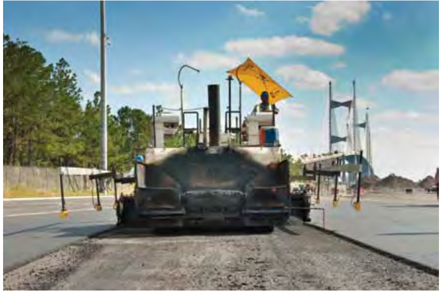
The Roadtec RP 185-10R paver was equipped with dual averaging skis and six Trimble ST200 sonic tracers (three on each side) to match asphalt slope requirements to the drain gates.
