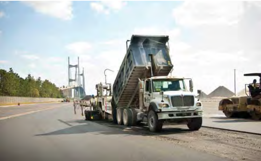
The Trimble PCS400 allowed Yates to further fine tune slope requirements and deliver a warranty project not many contractors would consider.
